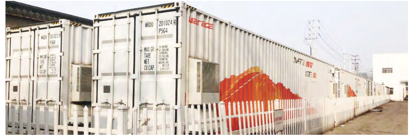
7MW/30MWh, C&I ES project, Jiangsu, China
