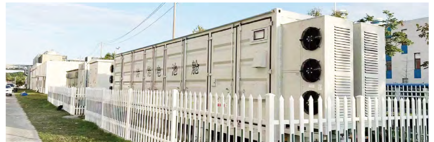
3MW/6MWh, C&I ES project, China
