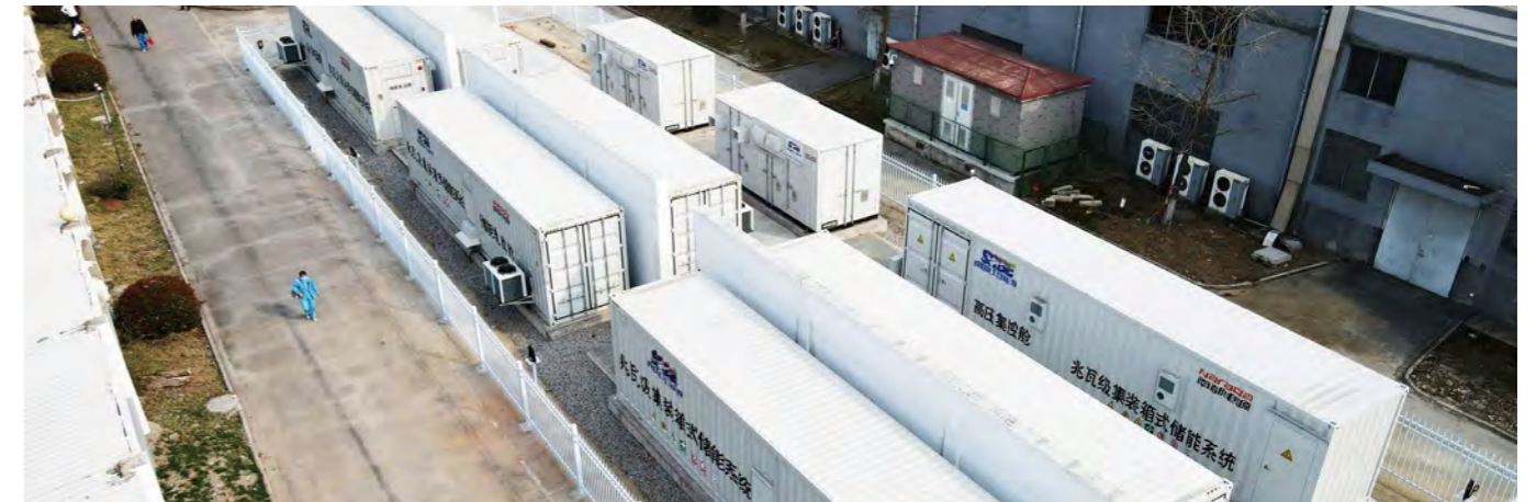
3.75MW/15MWh, C&I ES project, China
