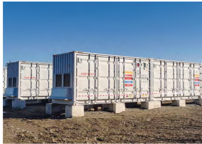
70MW/340MWh, frequency regulation, Italy
