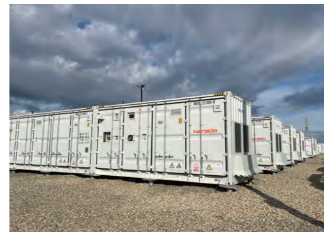
71MW/129MWh, PV+ESS, USA
