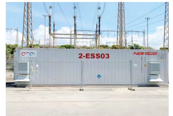
22MW/22MWh, thermal plant AGC frequency regulation, Italy
