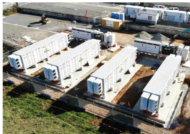
10MW/20MWh, frequency regulation, Australia
