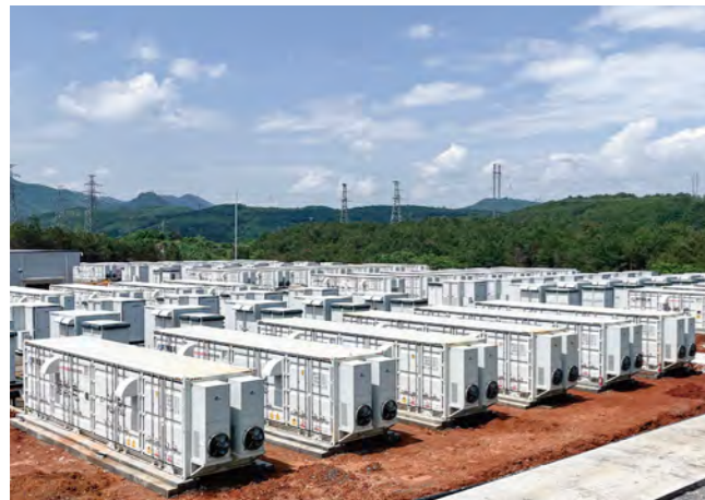
100MW/200MWh, frequency regulation, Hunan, China
