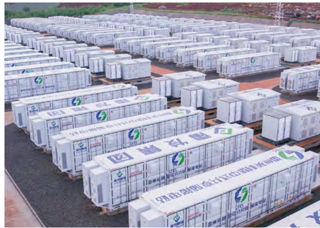
200MW/400MWh, frequency regulation, Guangdong, China
