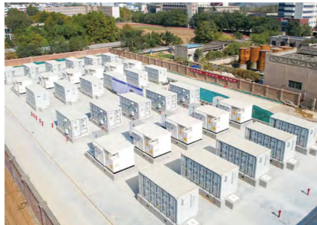
100MW/200MWh, frequency regulation, Henan, China
