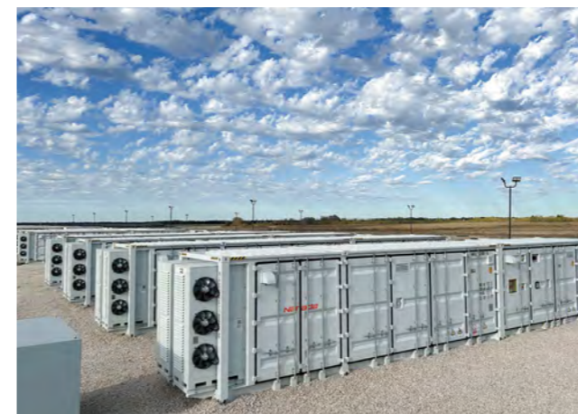
71MW/129MWh, PV+ ESS, USA
