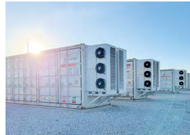
71MW/130MWh, wind+ ESS, Texas, USA
