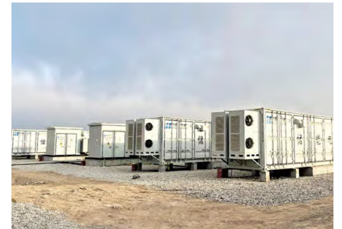
60MW/125MWh, PV+ESS, Xinjiang, China
